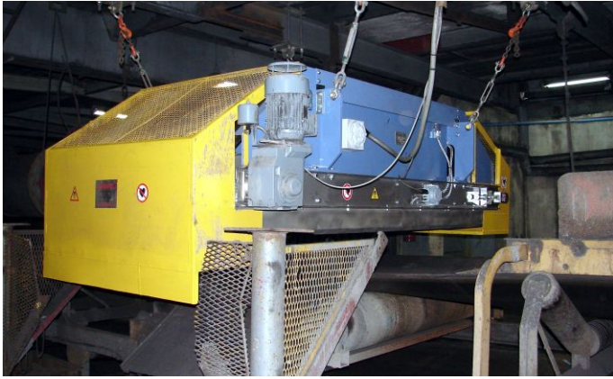
Removal of tramp iron from coal.
