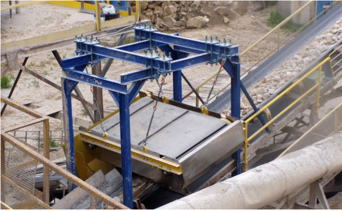
Protection of lime stone crusher against tramp iron.
