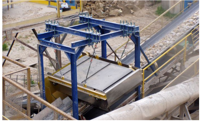
Protection of the limestone crusher against tramp iron.
